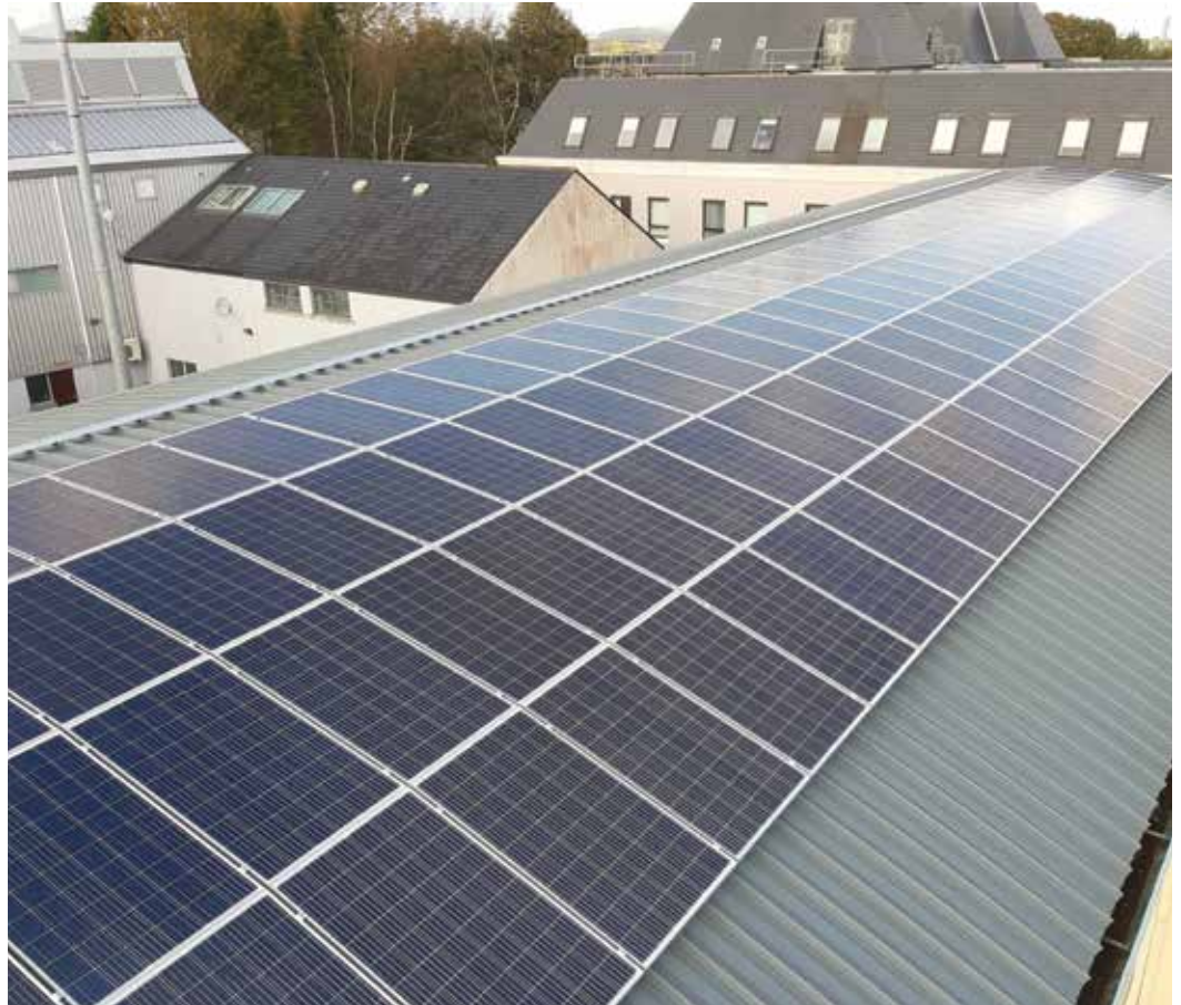
Mayo County Council has installed an 84kW solar PV array on Aras an Chontae, Castlebar. The 301 PV panels will provide over 11% of Aras an Chontae's electricity usage and will offset over 30,000kg of CO 2 per year.
