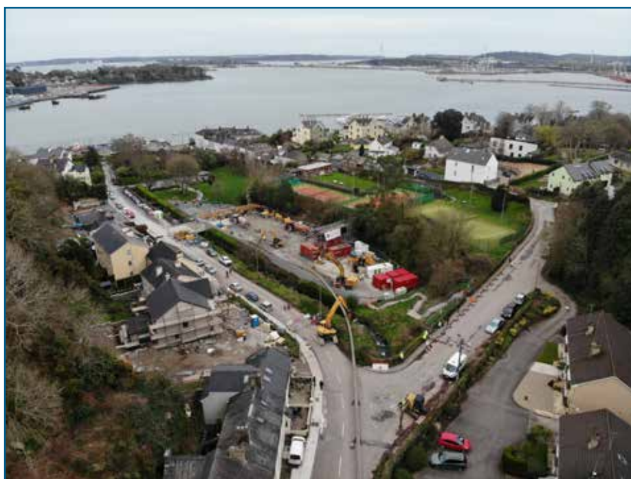
Pipeline installation as part of the longest horizontal directional drill on the Cork Lower Harbour Main Drainage Project.
