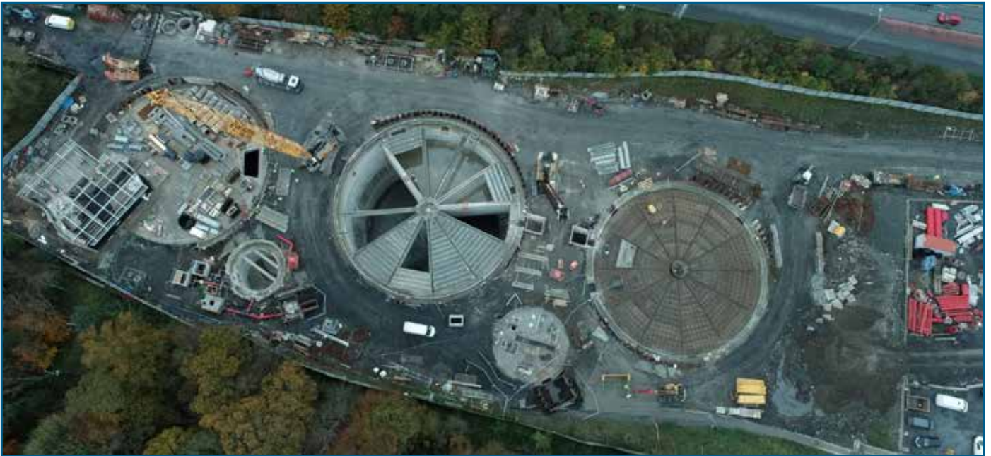
Construction of the three main storage tanks (30,000m 3 ) on the Blanchardstown Regional Drainage Scheme (BRDS).
