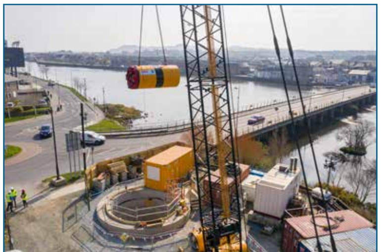
Mobilising a Tunnel Boring Machine (TBM) at one of the many trenchless shafts for the Arklow Wastewater Treatment Plant Scheme.
